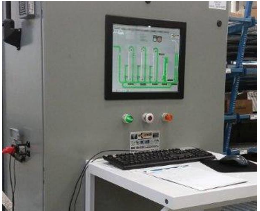
Control Design & Build by Top Shelf Team
